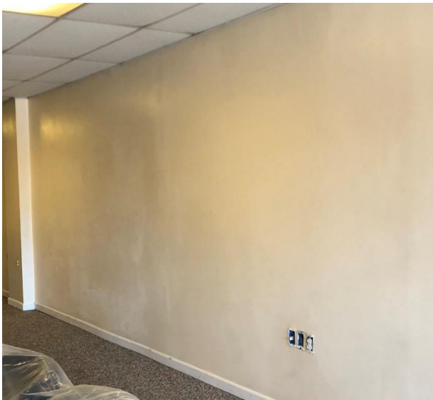
The back wall is an off-white. Yes, that spot that appears to need some touch-up paint did receive more paint.
